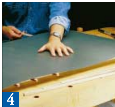
4 Starting at the center of the panel, remove the spacers and press the laminate down. The contact cement will bond instantly.
