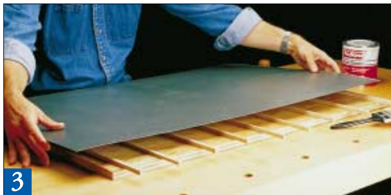
3 After you apply contact cement to both the laminate and substrate and let it dry, set clean spacers onto the substrate. Then position the laminate roughly in place.
