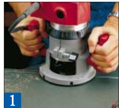
1 With the rough size marked on the face of the laminate, support the material near the line and rout it with a straight bit.
